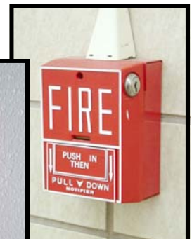
Fire Alarm Pull Station
