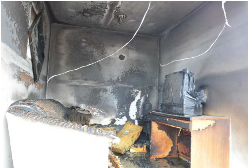
This room had no sprinkler.
