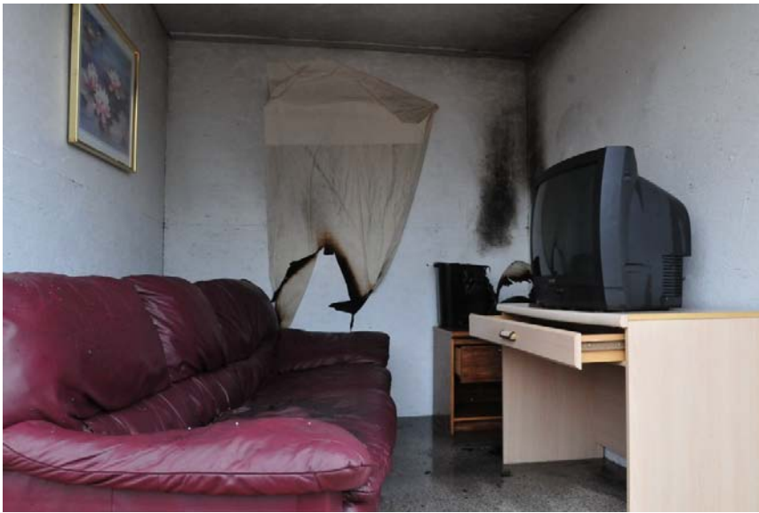
This room DID have a sprinkler.
