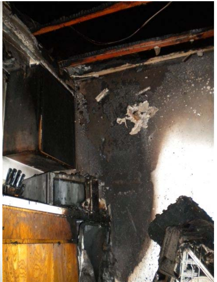
Inside the kitchen, damage is extensive and the roof is completely gone.
