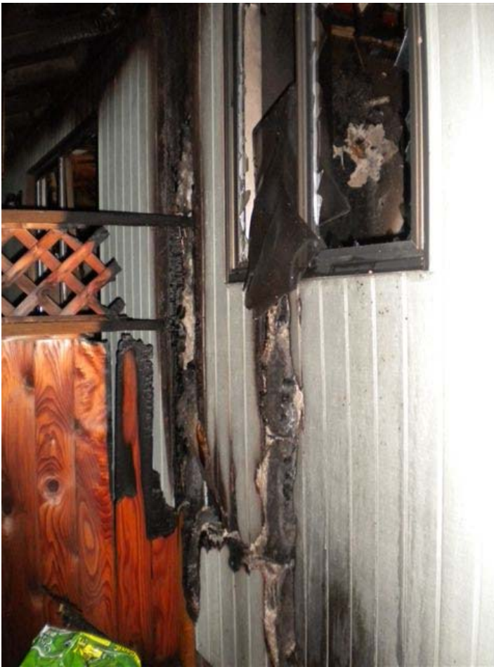
The exterior wall adjacent the kitchen where it's believed this fire started.
