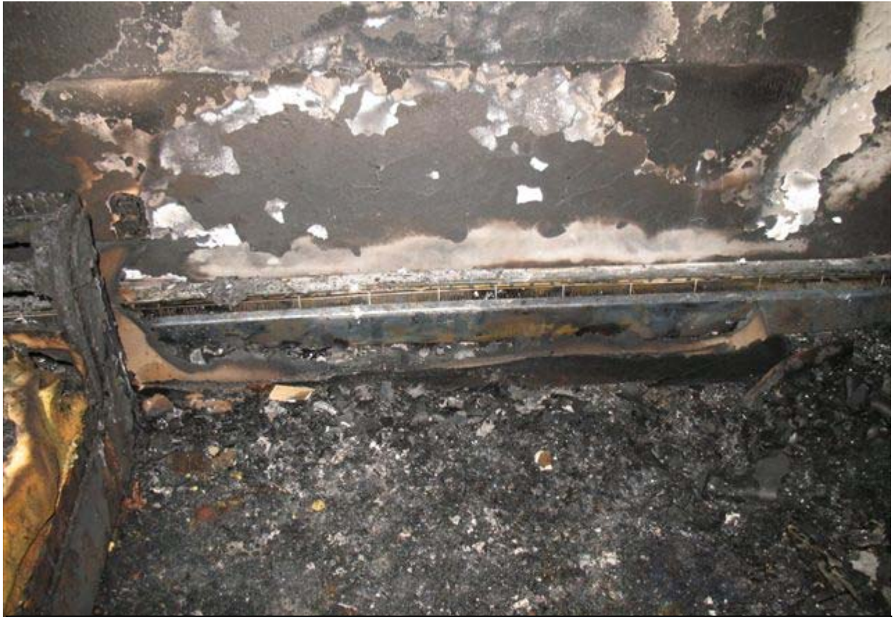
This fire was the result of combustibles placed too close to an electric baseboard heater.
